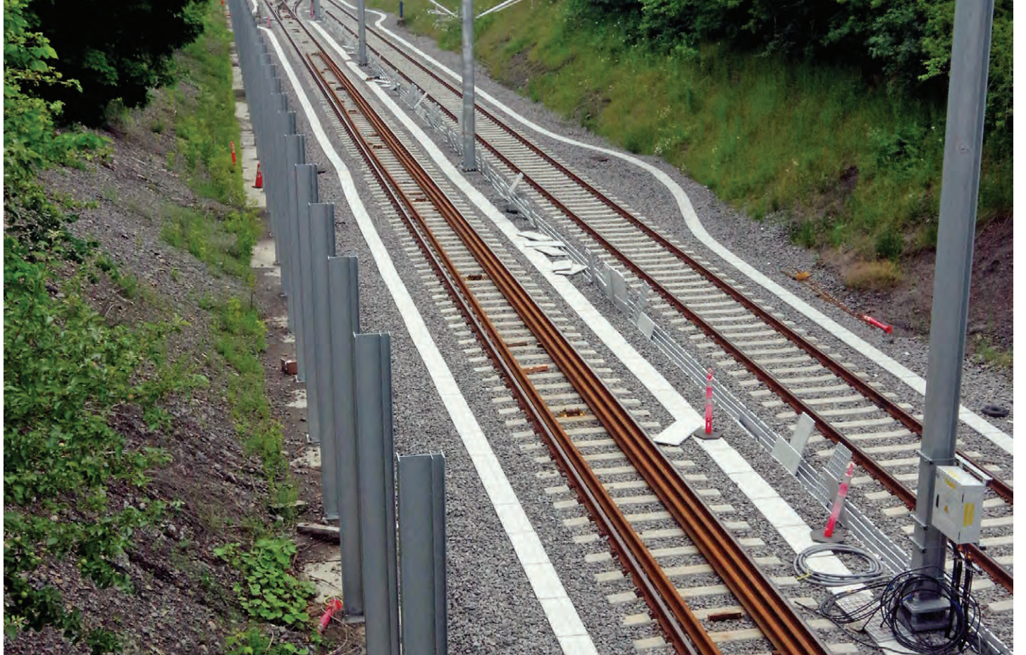
While there are no trains yet along the REM line which travels south to north across the centre of TMR, initial reports from other areas of Montreal suggest the trains are noisier than the developer, CDPQ Infra, has claimed.
